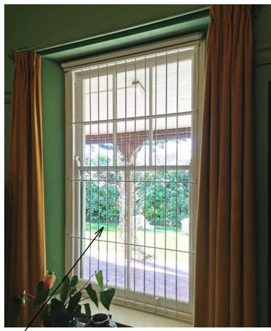
typical sash window - single glazing with inadequate burglar bars
