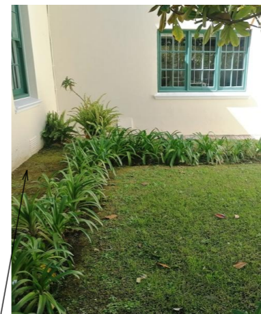
soil levels too high in relation to the internal floor levels
