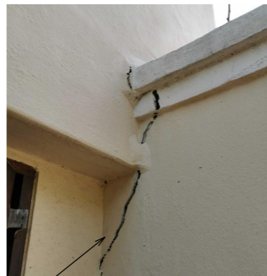
Severe structural cracking between gate pillars and coach house and Museum.
