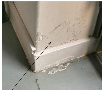
damp to the walls in the outbuildings where the exterior ground levels are too high
