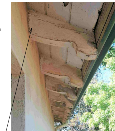
Eave sprockets, fascias and soffits to be repaired/replaced & painted
