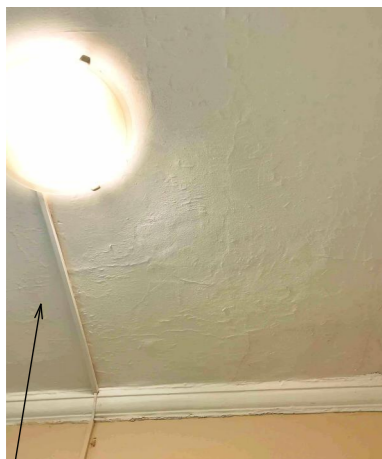
Plasterboard ceiling & cornice in passage in poor condition to be repaired / replaced with all services hidden
