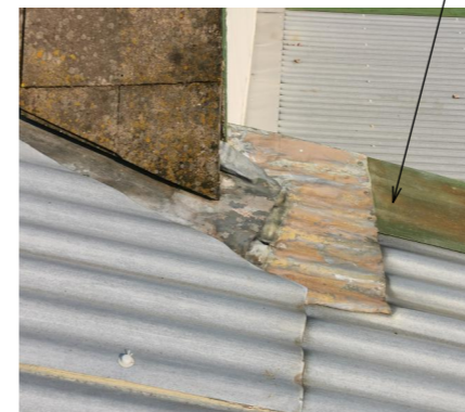
roof repairs done with mixture of new & old materials- all to be replaced
