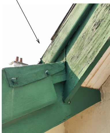
Roof junctions between different roof finishes (asbestos tile and corrugated iron) require regular maintenance and careful restoration
