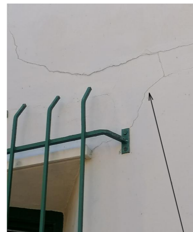
example of external plaster & structural cracks
