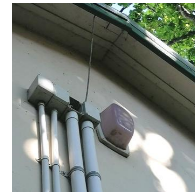
Multiple external surface mounted conduits
