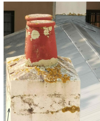
poor maintenance to the chimneys allows water ingress into the walls & structure below
