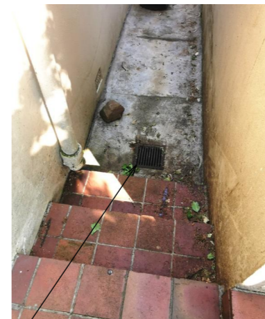
Single outlet point in service alley risk of flooding if blocked
