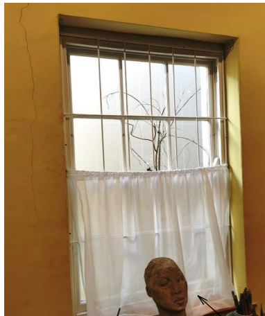
West facing window in Irma's Studio, UV and light levels concerning
