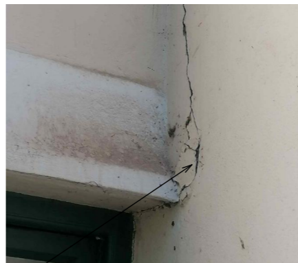
Cracks in the walls to Irma's Studio
