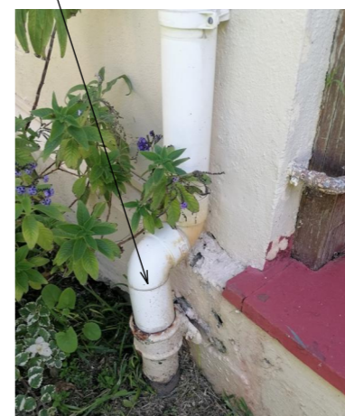
generally the down-pipes & storm water disposal needs to be upgraded to avoid excess moisture around the structures
