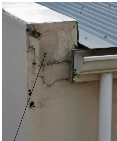
parapets require maintenance & upgrading
