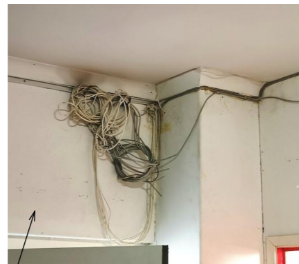
Store 1- multiple & redundant cables for data & other services are poorly installed and can not easily be maintained in the current layout
