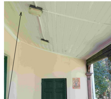
curved timber ceiling to verandah to be redone when restoring / repairing the roof & structure
