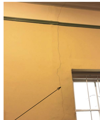
structural cracks through walls will allow water ingress & damp into the interior
