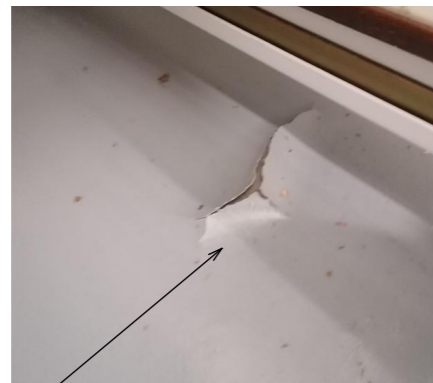
Epoxy floor failing in Store 2 & Kitchen
