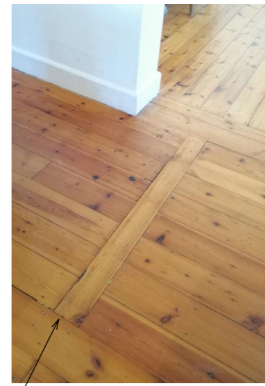
Patchwork repairs to first floors
