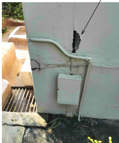
cracks, damaged plaster & poor service installation allowing ingress of water
