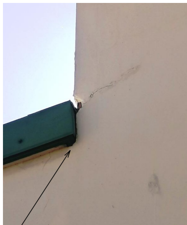
poor plaster works and flashing at roof junction
