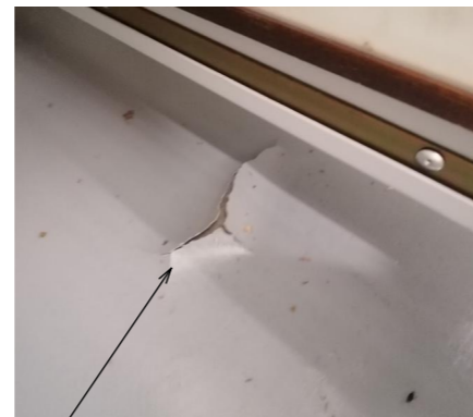
Failing epoxy finish to floor in Store 2
