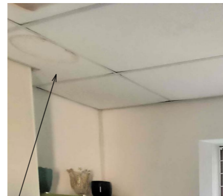
Kitchen ceiling tiles damaged
