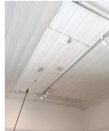
uncoordinated layout of lighting, alarm & fire installations to the 1st floor degrade the ceilings
