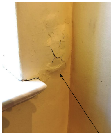
spalling plaster internally on stairwell
