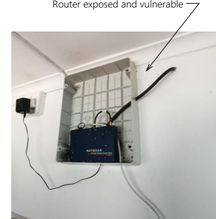
Router exposed and vulnerable
