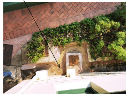
Rainwater channel clashing with drainage.
