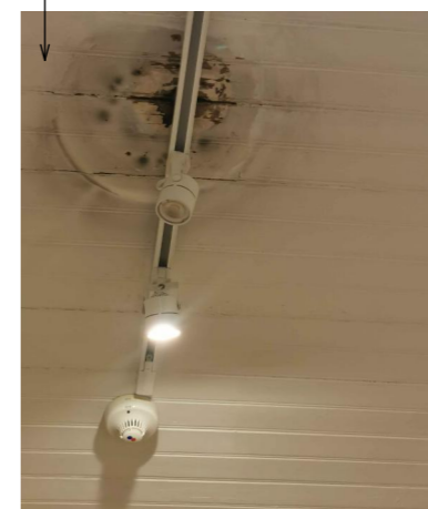
Gnd Floor - T&G ceilings to be restored & services rationalised
