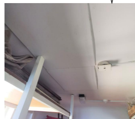
Plasterboard ceiling in Store poorly patched, to be replaced
