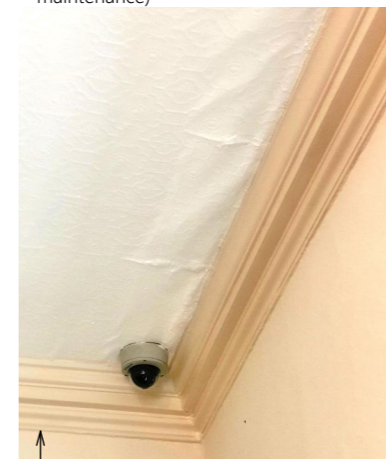
(Dining Room) Embossed wallpaper coming loose, to be restored or replaced to match
