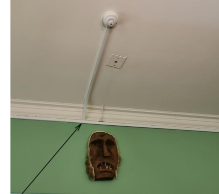
Unsightly surface mounted trunking and exposed wiring.
