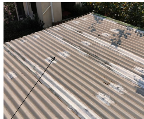
Unpainted galvanised corrugated roof sheeting in fair condition can be retained with minor repairs & maintenance
