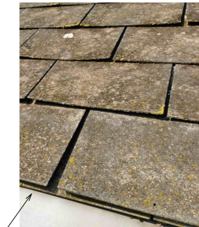
Asbestos roof tiles irreparable
