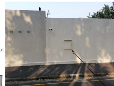
Municipal electrical box on Cecil Street vulnerable to vandalism
