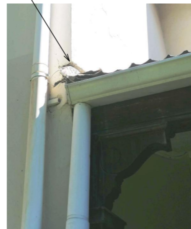
poor installation of roof flashing & counterflashings
