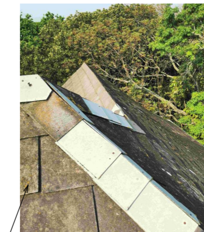
Asbestos roof tiles: all tiles are extremely brittle, curved with fixings coming loose
