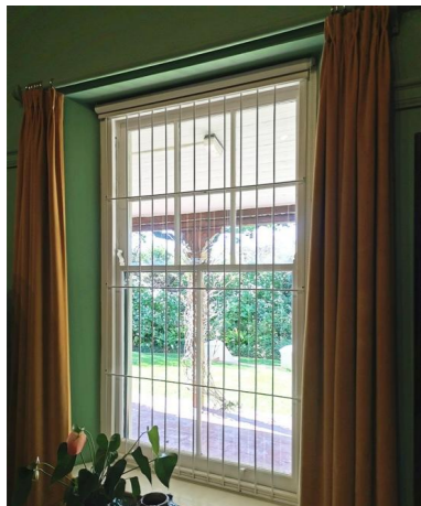
Opening windows not suitable for environmental control
