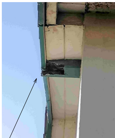
All rotten timbers to be replaced NB structural members as above
