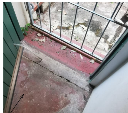
Store 1 door with no doorsill to outside or waterproofing- water free to travel under door to interior
