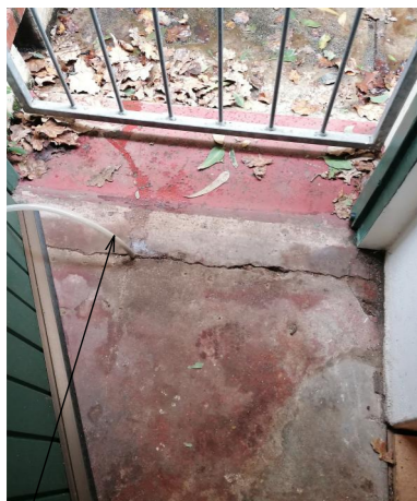
External access into Store 1 is very insecure, vulnerable to the environment & water ingress. Floor visibly damp
