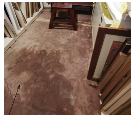
Store 1 floor screed cracked, damp, no dpm
