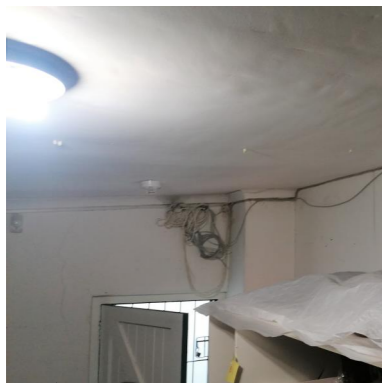
Store 1: Plasterboard ceiling damaged and sagging possibly due to water ingress. Note surface wiring and services!
