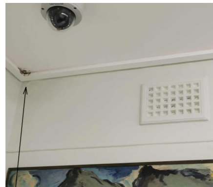
Store 2 hole in ceiling
