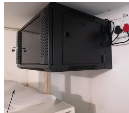
Server unit in Store 1 poorly installed, propped up on the shelving unit. Required routine maintenance will grant service agents access to the archive
