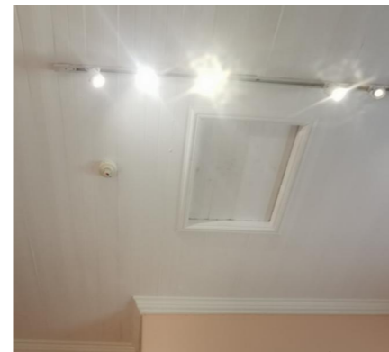
Data connection exposed and vulnerable
