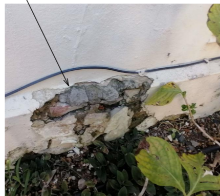
crumbling brickwork to substructure
